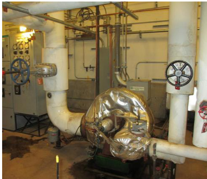
Cordwood energy system (photo by David Nicholls)
